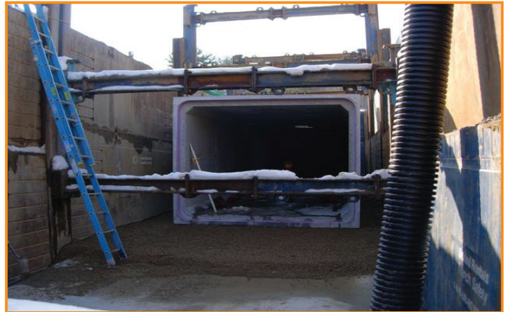
Linear system used for a large vault
